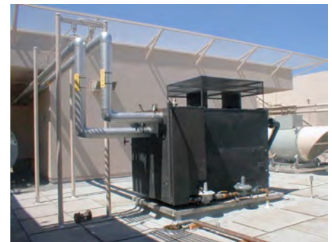
Rooftop installation of T1995LR 12PPM 85% eff. outdoor model hot water boiler at the Lakeshore Towers.
