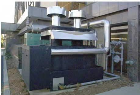
1st Tennessee Bank in Johnson City, Tennessee has a T2970 Direct Fired Hot Water Boiler installed outdoors.
