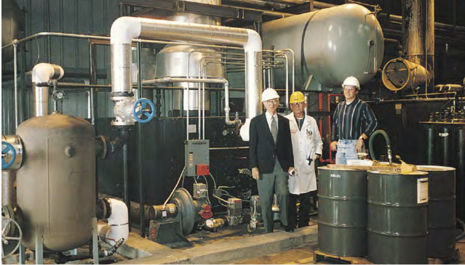
Installation of more than ten Parker Steam & Thermal Fluid Heaters in various locations at PRC-Desoto International Courtaulds Aerospace in Mojave, CA.
